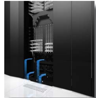
More efficient cooling through improved airflow
