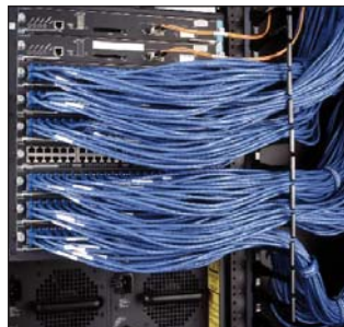
Figure 7 – Cables on front of Cisco switch
