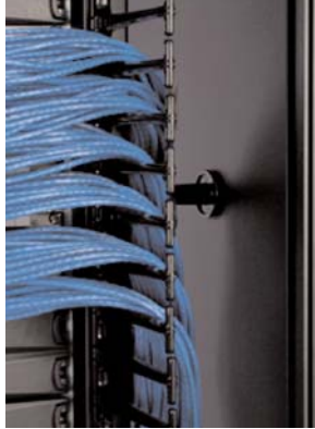
Figure 9 – Cable management inside cabinet
